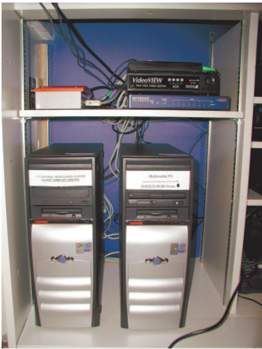
Sunny Boy photovoltaic control hardware, video splitter, keyboard/monitor switch, Netgear router/firewall, two Compaq PCs.
