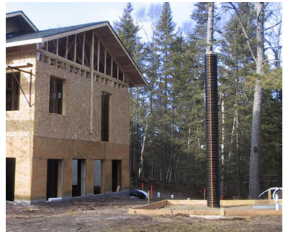
The pier as it appeared all winter. It is 16 foot high and 16" in diameter. It extends up 4' from an underground to underground 8x10 foot base so is 20 foot tall in total. A 2 foot steel pier was later attached to that.
