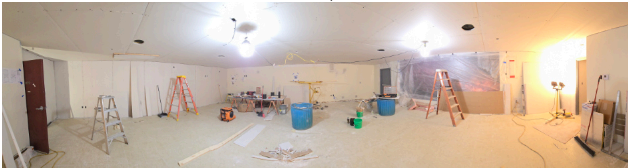
Below: panoramic view looking north. All drywall installed as of February 6 th .
